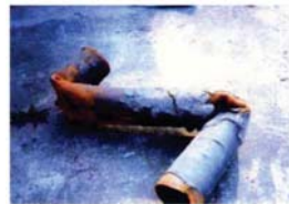
Photo 2 Damaged gas pipeline at Wu Xi Bridge in Taiwan
