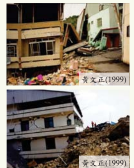
Building failure caused by reverse faulting
